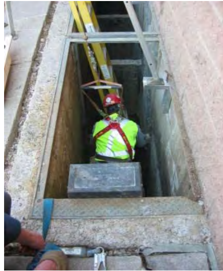
Even if the entry is not under confined space rules, the tripod and harness may be required for fall protection.
