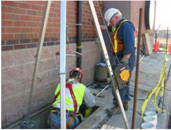
Note the brackets on the side wall temporarily installed for the tripod.
